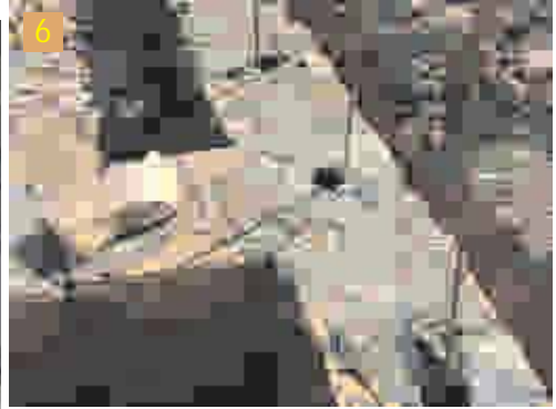
Pull out the pipe and fill up the cavity with 1:1½:3 micro concrete for Zone IV & V and 1:2:4 micro concrete for Zone III while continuously rodding. Ensure min. 50mm (2") concrete all around the bar. Put back pipe in place and continue with masonry construction around it.
