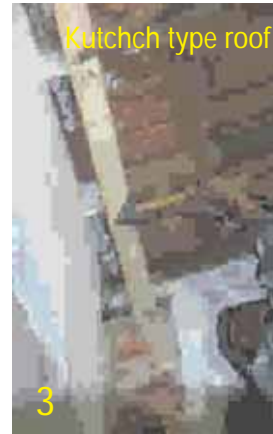
3. Using two nails at each end install a 100mm (4") x 25mm (1") strut (plank) on the underside of the rafters adjacent to their both ends.
