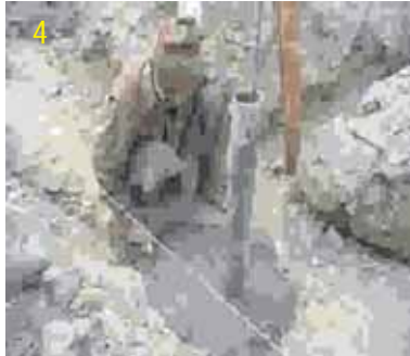
Insert 100mm (4") diameter PVC pipe 900mm (36") long over all vertical reinforcement bars.
