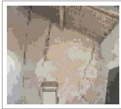
Moderate and fine cracks
