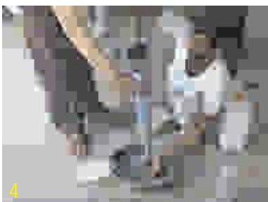
4. Fill up hydraulic pump or a simple hand-pump with non-shrink cement slurry.
