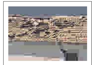
Roof distortion damage
