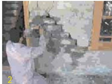
2. Fix grouting nipples in the 'V' groove at a spacing of 150mm to 200mm, or leave holes at that spacing while sealing the crack with 1:3 cement mortar.
