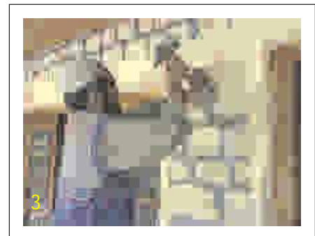
3. Rake all the mortar joints to the depth of 12mm (1/2") by chisel or electric grinder. Clean the surface with wire brush.
