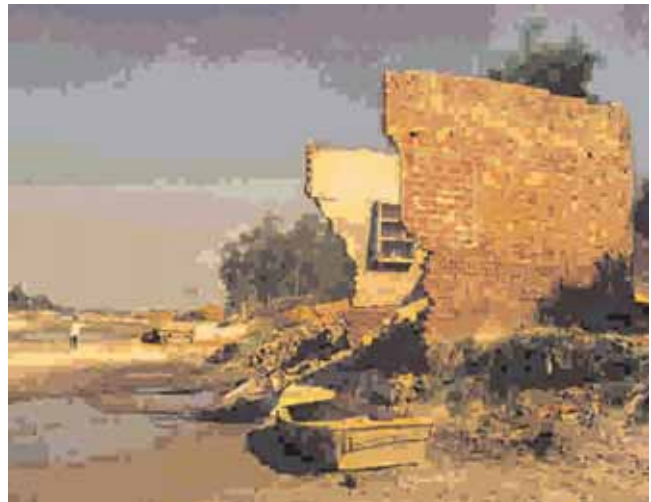
Wall collapse due to tidal surge
