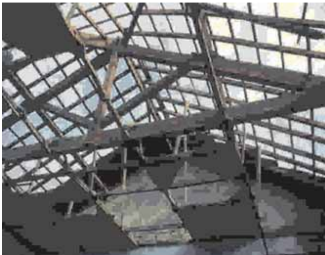
Blown off tiles due to high winds
