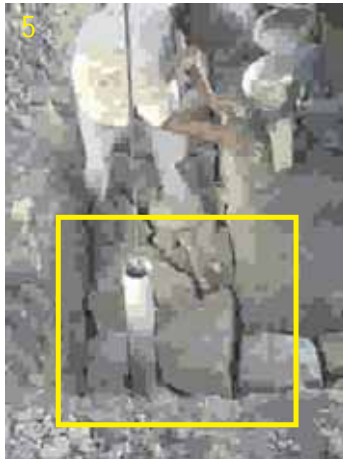
Construct stone masonry up to 450mm (18") height keeping pipe piece in place.
