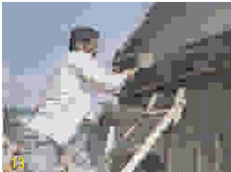
13. Splash the exposed wall surface with water and apply neat cement slurry followed by first coat of cement : sand (1:3) plaster.
