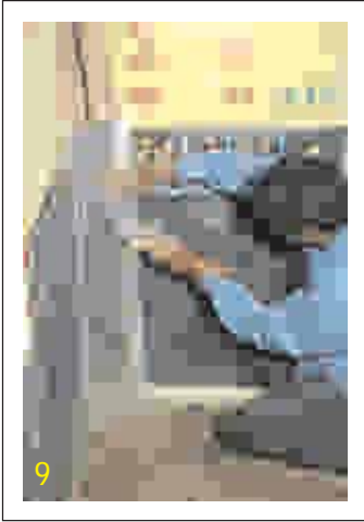
9. Once all the shear connectors are grouted, clean the wall with wire brush and water. Install GI or timber centering for concreting.
