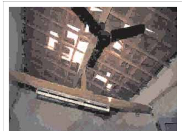
Roof Tiles blown off
