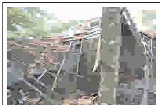
Wall & Roof damage by Cyclone
