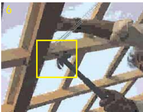
6. Tie one wire at a time around the joint of strut with rafter or purlin, stretched with carpenter's hammer.
